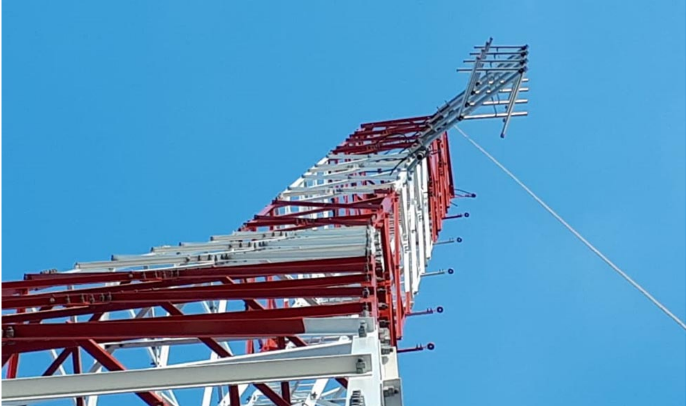
The aerial on the top of the tower has been perfectly positioned.
