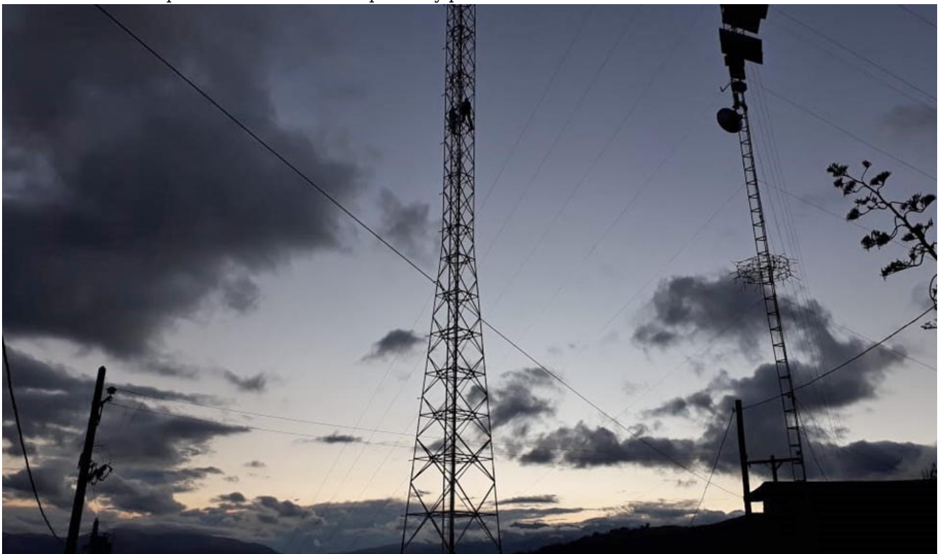
Night quickly comes upon us. Two workers of Diospi Suyana are working frantically in the tower (see middle of the picture).
