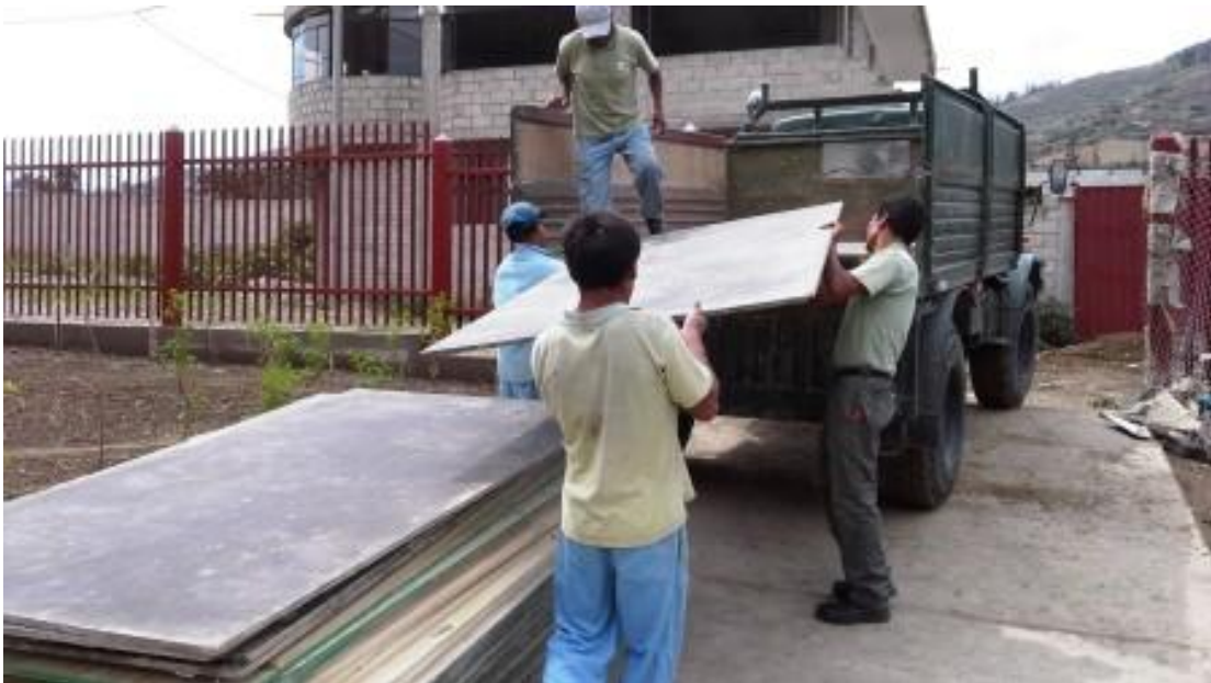
The form panels are no longer needed at the school, but will certainly be used at the next construction location.
